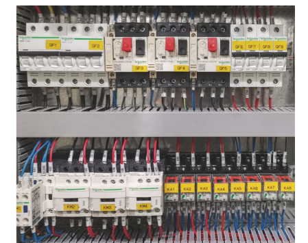
SCHNEIDER electricity parts
